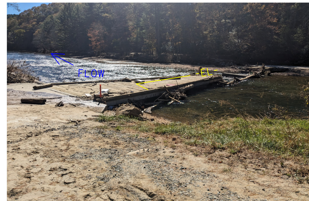
PHOTO #4: UPSTREAM OF DAMAGED EXISTING BRIDGE.
